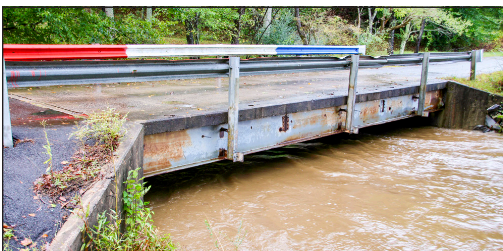
County officials kept a close watch over the Byers Road bridge during Tropical Storm Helene. Thankfully, the bridge did not flood as the county continues to work on a solution for those one-way in and out neighborhoods. Photo by Shawn Jarrard
