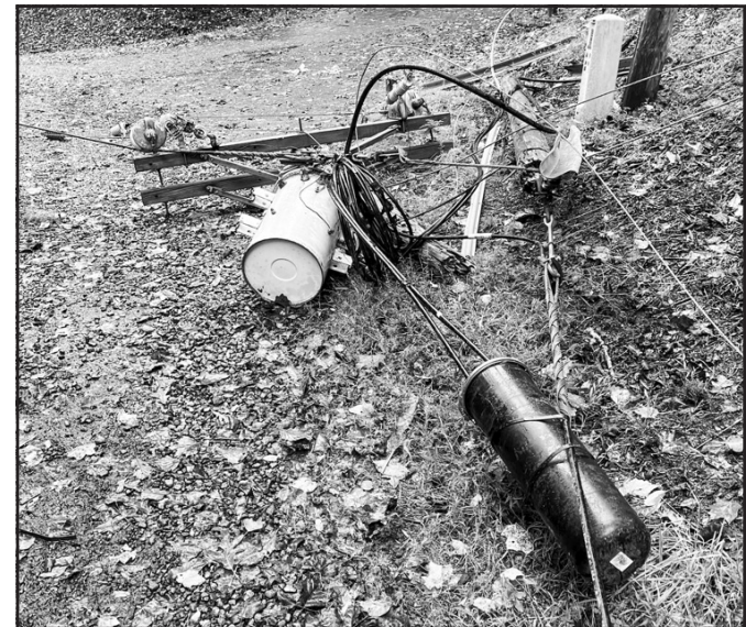
Blue Ridge Mountain EMC restored power quickly over the weekend after Tropical Storm Helene, having to replace just eight power poles systemwide.
